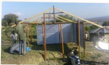
CONSTRUCTING NEW WASHING ROOMS AT THE KAMIN ONINGO FISHING BEACH IN KENYA.
