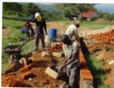
WORKMEN PREPARE THE BASE OF TWO NEW CLASSROOMS AT THE BUSAGAZI SCHOOL IN UGANDA
