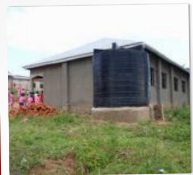
WATER TANK INSTALLED BY CANASSIST AT THE KAYENJE SCHOOL IN UGANDA.
