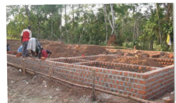
WORKERS BUILDING TEACHERS' ACCOMMODATION WITH CANASSIST FUNDING AT THE HOPE FOR YOUTH SCHOOL.
